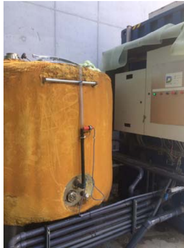
Figure 6. Adding an extra buffer tank to work in a continuous way. The liquid fraction of the digestate is continuously refreshed while the installation continues with the stripping and scrubbing process.
